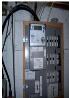
The image above shows a "smart meter" in an industrial building.
