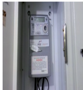
The image above is a "smart meter" in an office.
